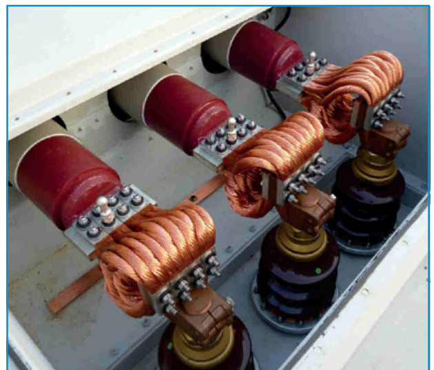
Copper braids to transformer
