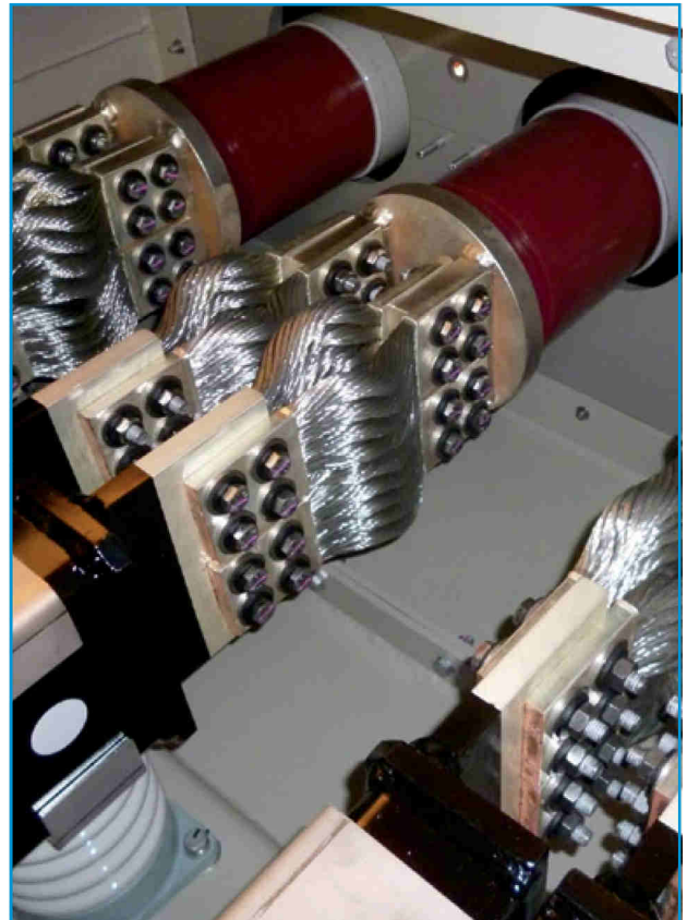
5000A generator connection
