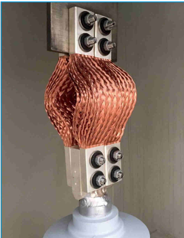
Copper braids to transformer
