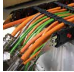
Program LC55: Wired with cables and connectors
